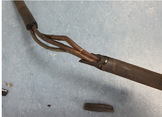
Figure 5: Part of the degraded cable sample
